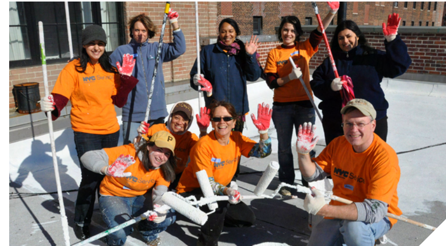
Employees donate their time to paint roofs reducing greenhouse gas emissions and energy usage.
